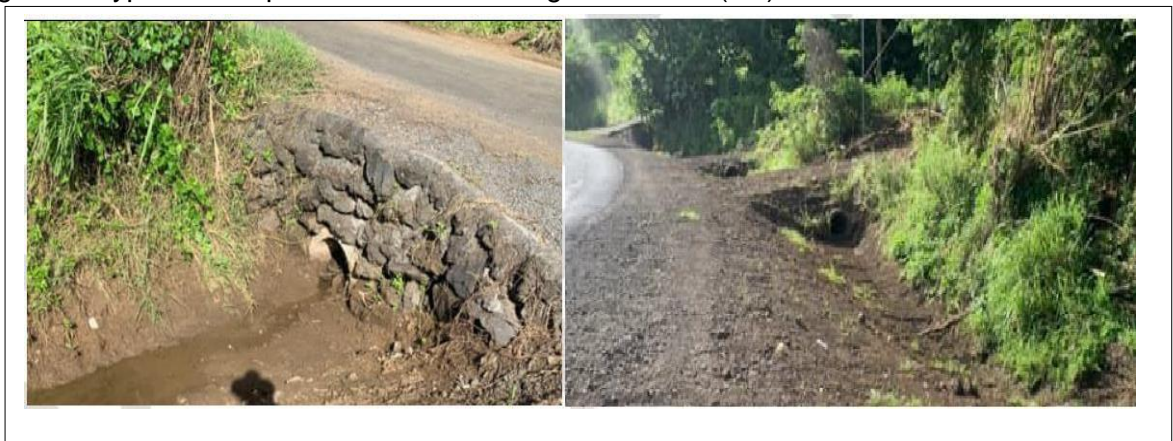
Figure 4: Typical examples of culvert crossing under road (left) and roadside swale drain
