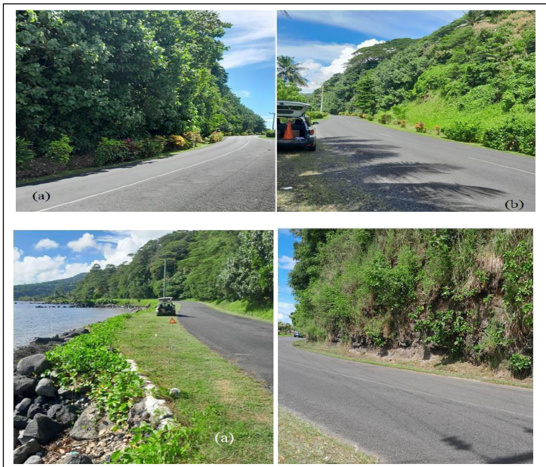
Figure 5: Views of the ECR showing steep rising slopes on the landward side.
